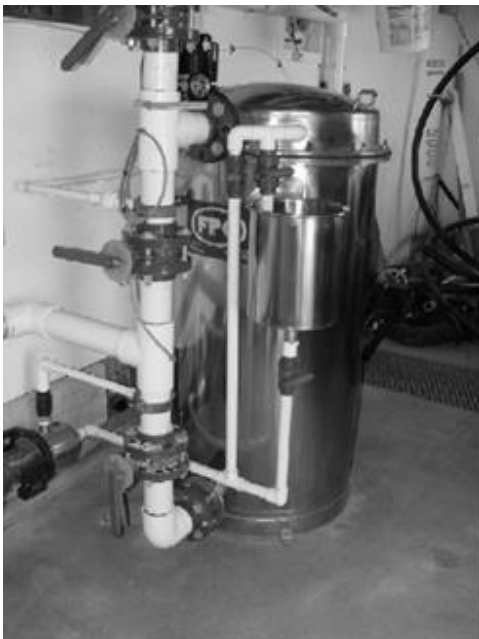
Figure 14.1: Diatomaceous earth pressure plant at Mokau, Waitomo District
