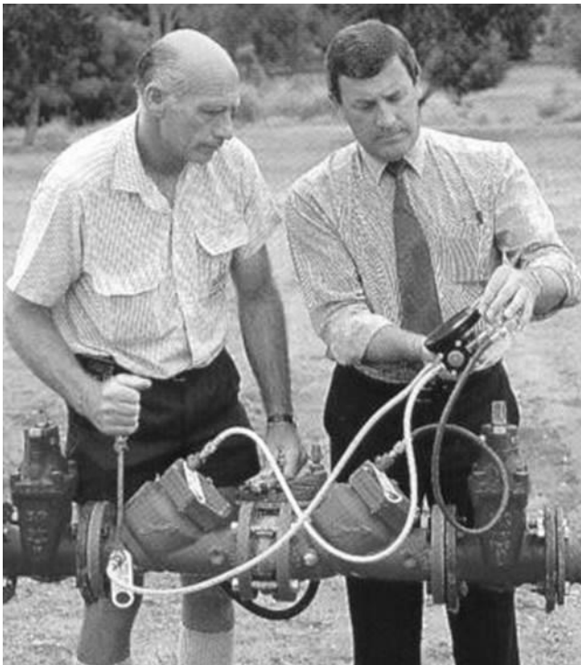
Figure 16.4: Commissioning a backflow prevention device
