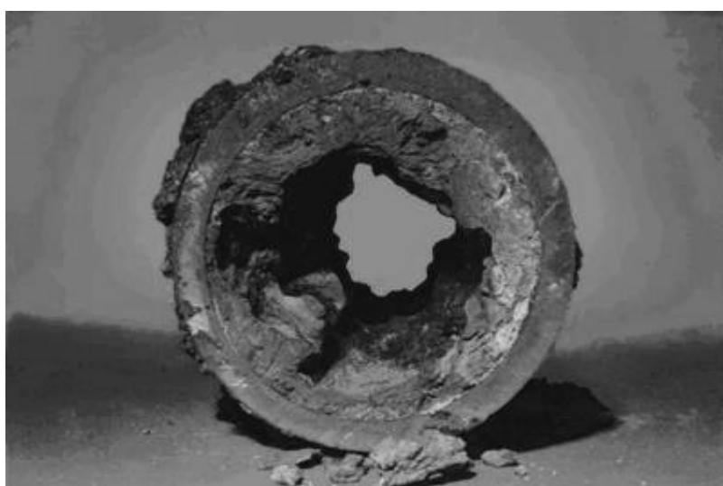
Figure 16.5: Example of corroded water pipe
